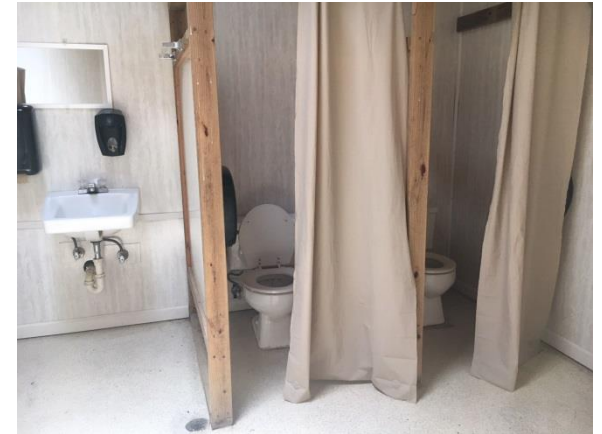
Indoor restroom facilities.
